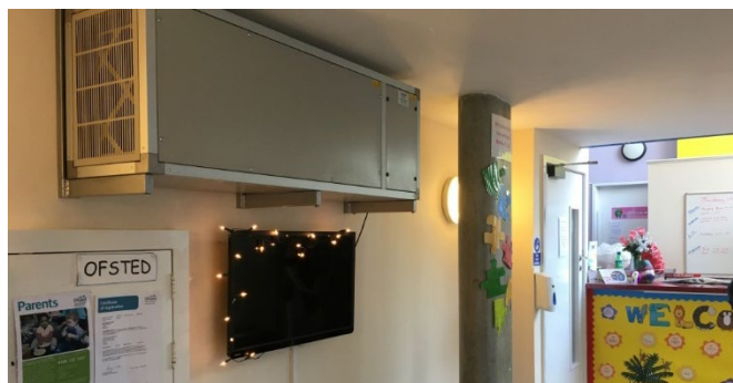
Picture 1 Recirculation Indoor Air Quality Filtration System
